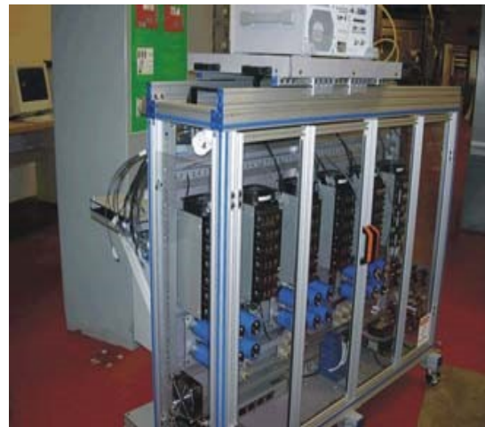
Mobile Power Electronics Rack
